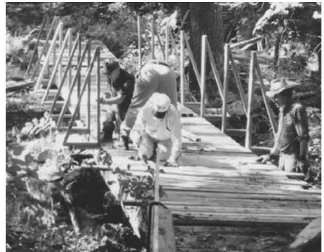
MidWeek Work Crew Redecking Broad Brook Bridge on Doolittle Trail Late in 2006
