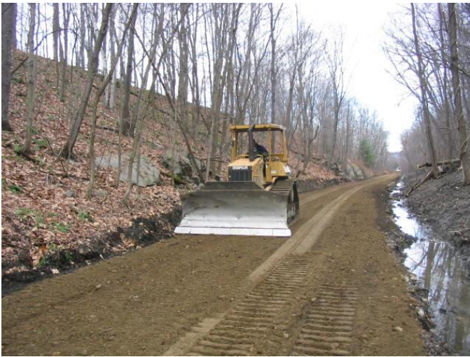
Grading the Improved Fort Hill Line Rail Trail. (Photo courtesy of Bill Roberts)
